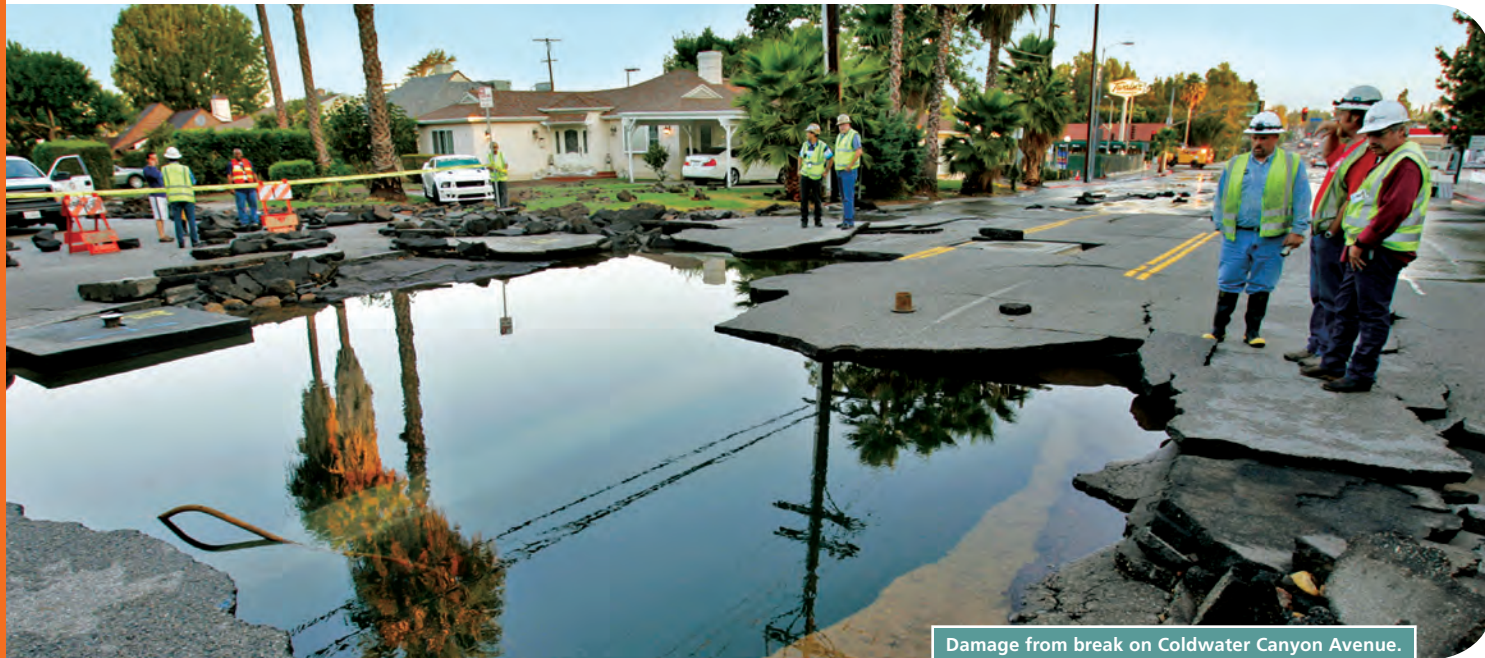
Damage from break on Coldwater Canyon Avenue.
